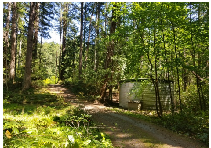
A 25,000 gallon water tank and several smaller tanks to be used for fire fighting and irrigation.
